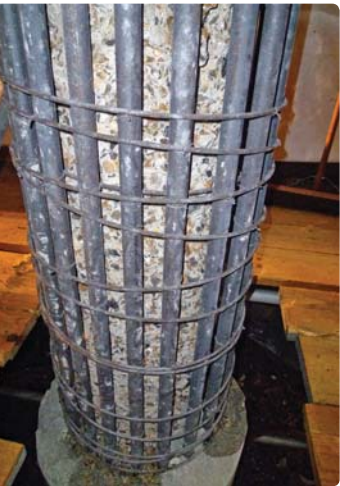
Figure 4: Column with defective concrete removed awaiting recasting.
