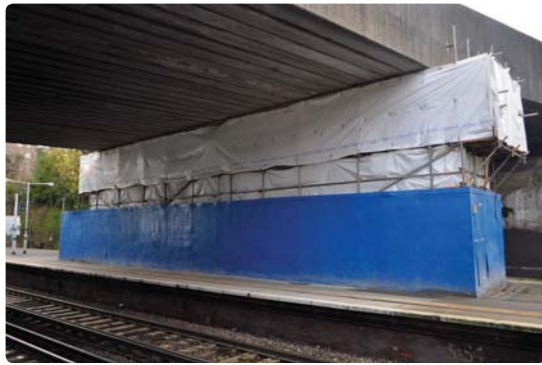
Figure 5 far right: Testing for shorts in the CP system prior to applying overlay with the spalled areas repaired and the beam prepared with the MMO titanium fabric and wiring ready to receive the overlay.
