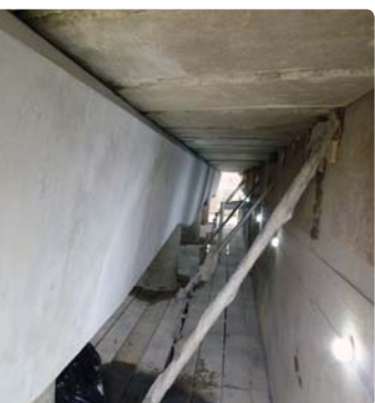
Figure 7 far right: The completed superstructure with new joints in place and re-asphalted.
